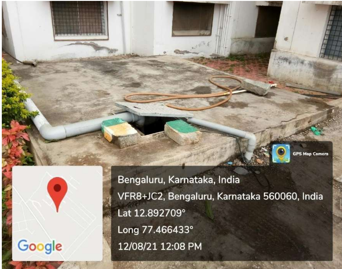
Photo: Tank to Store Rain Water
