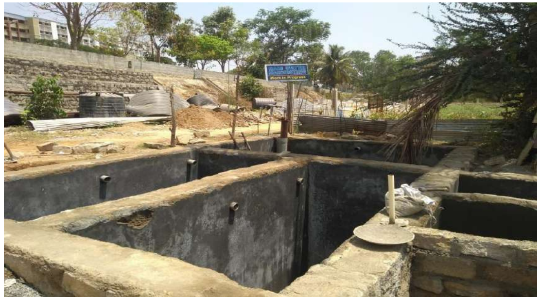
Photo: Rain water harvesting systems
