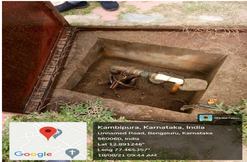
Photo: Borewell Recharge System in the Campus
