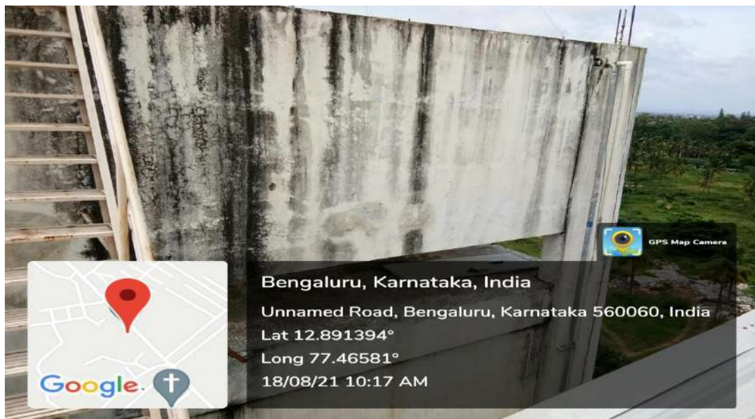
Photo: Over Head Tank in the campus building
