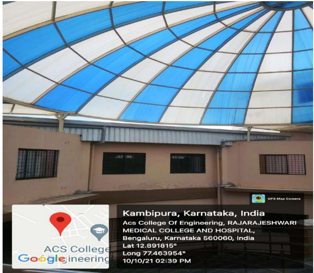
Photo: Roof Top Rain Water Harvesting
