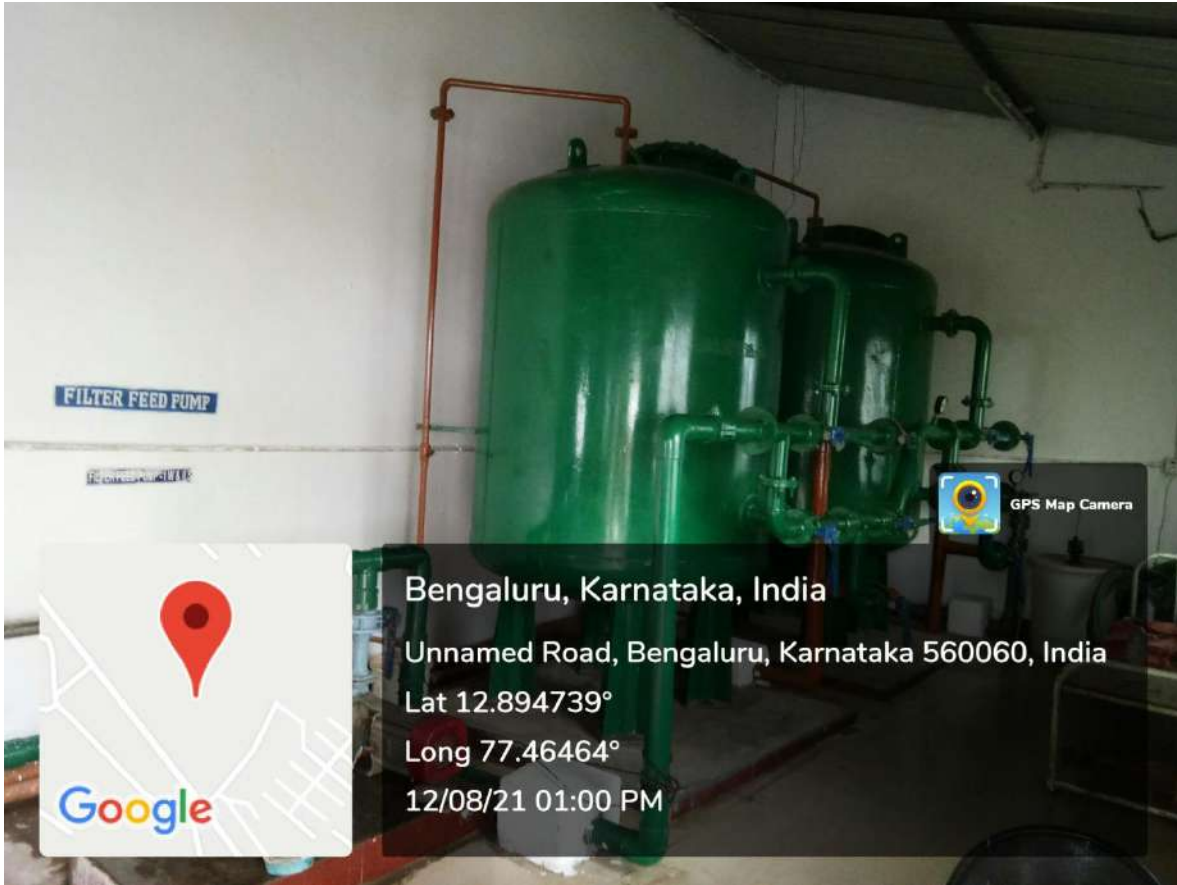
Photo: Sewage Treatment Plant in operation
