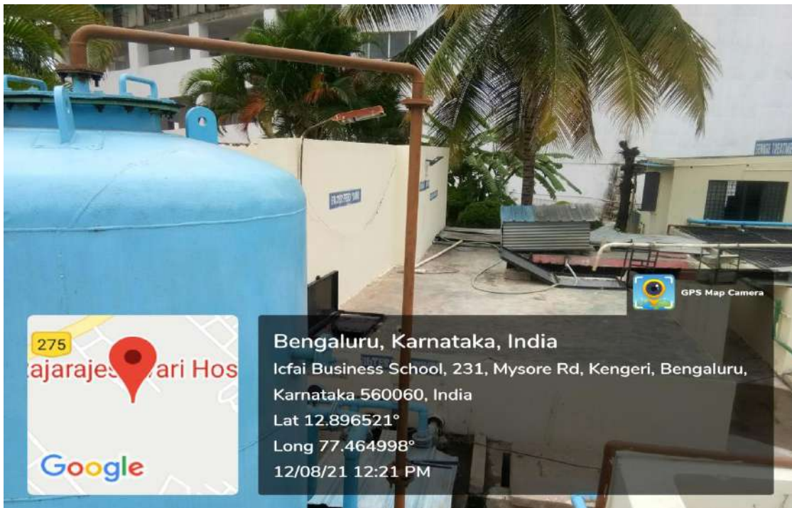
Photo: Sewage Treatment Plant
